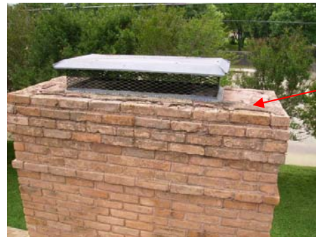
4 chimney cap erosion
