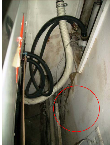
8 mold behind the washer
