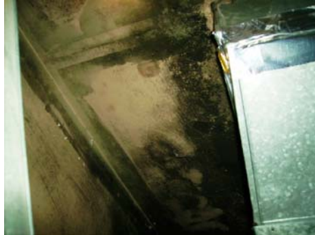
7 Looks like mold at furnace closet
