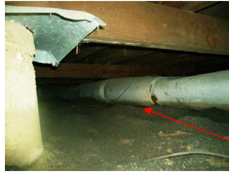
14 many rusting crawl space ducts
