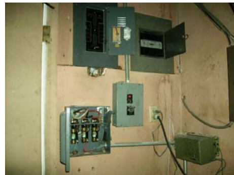
10 Advise review with electrician
