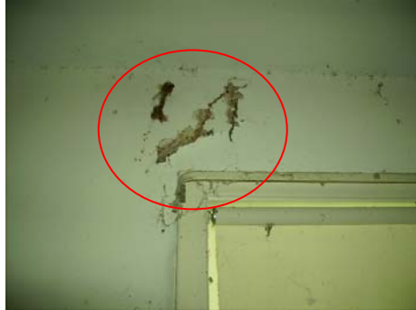
1 Termite evidence garage
