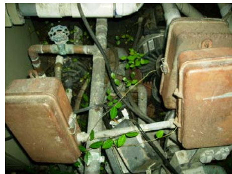
6 spa motor pump out (hard to see)
