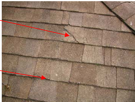
3 areas of roof shingle abrasion
