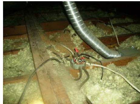
12 in the attic at least 10 electrical conditions noted
