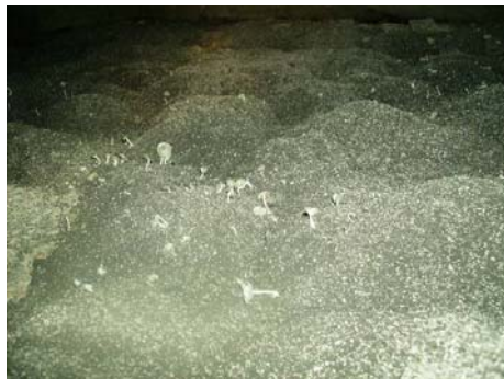
17 damp condition - mushrooms growing in crawl space
