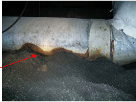
13 Rusted ductwork contacting earth
