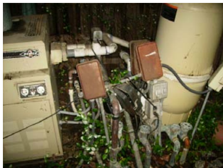
5 pool equipment - electrical hazard
